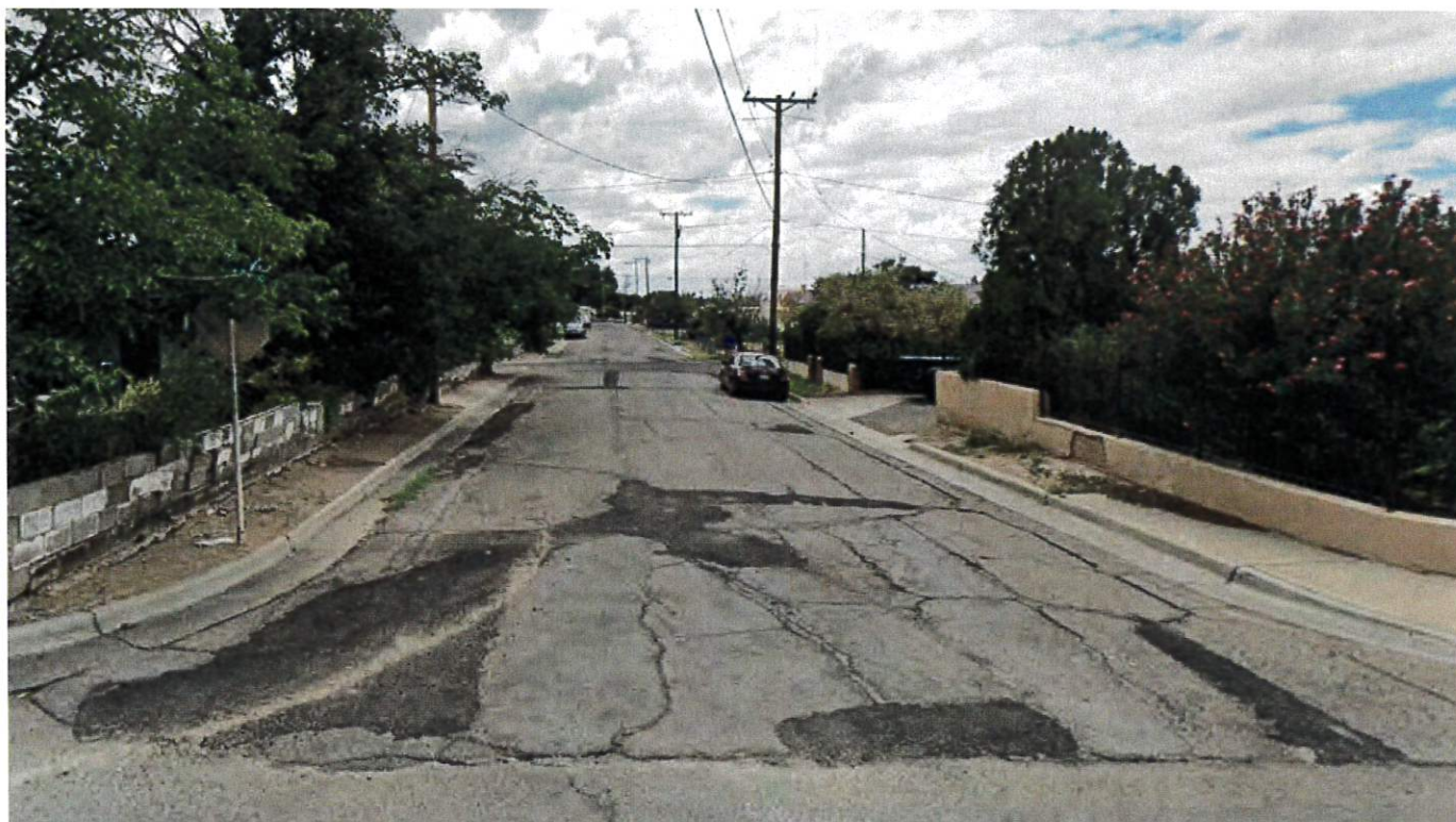
Appendix Image 7. Sidewalk gaps and deteriorating pavement conditions along Montana Ave.
