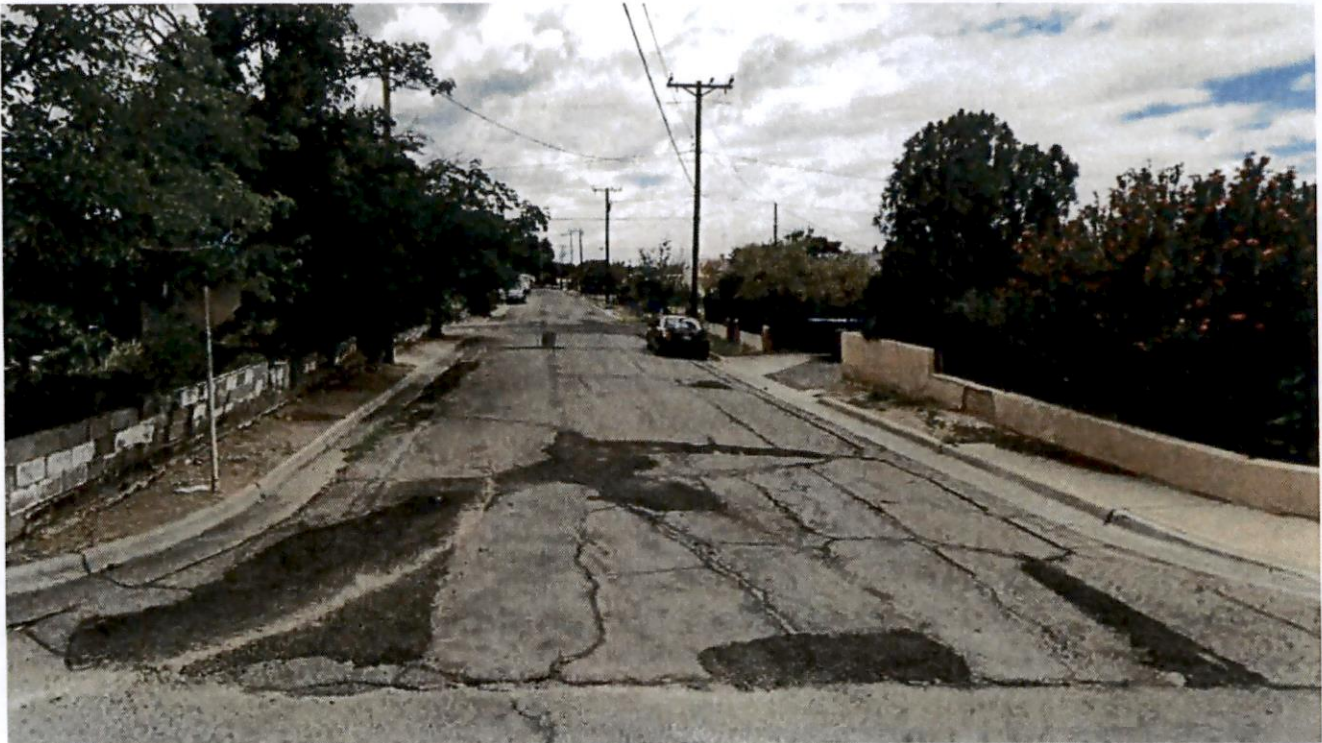
Appendix Image 7. Sidewalk gaps and deteriorating pavement conditions along Montana Ave.
