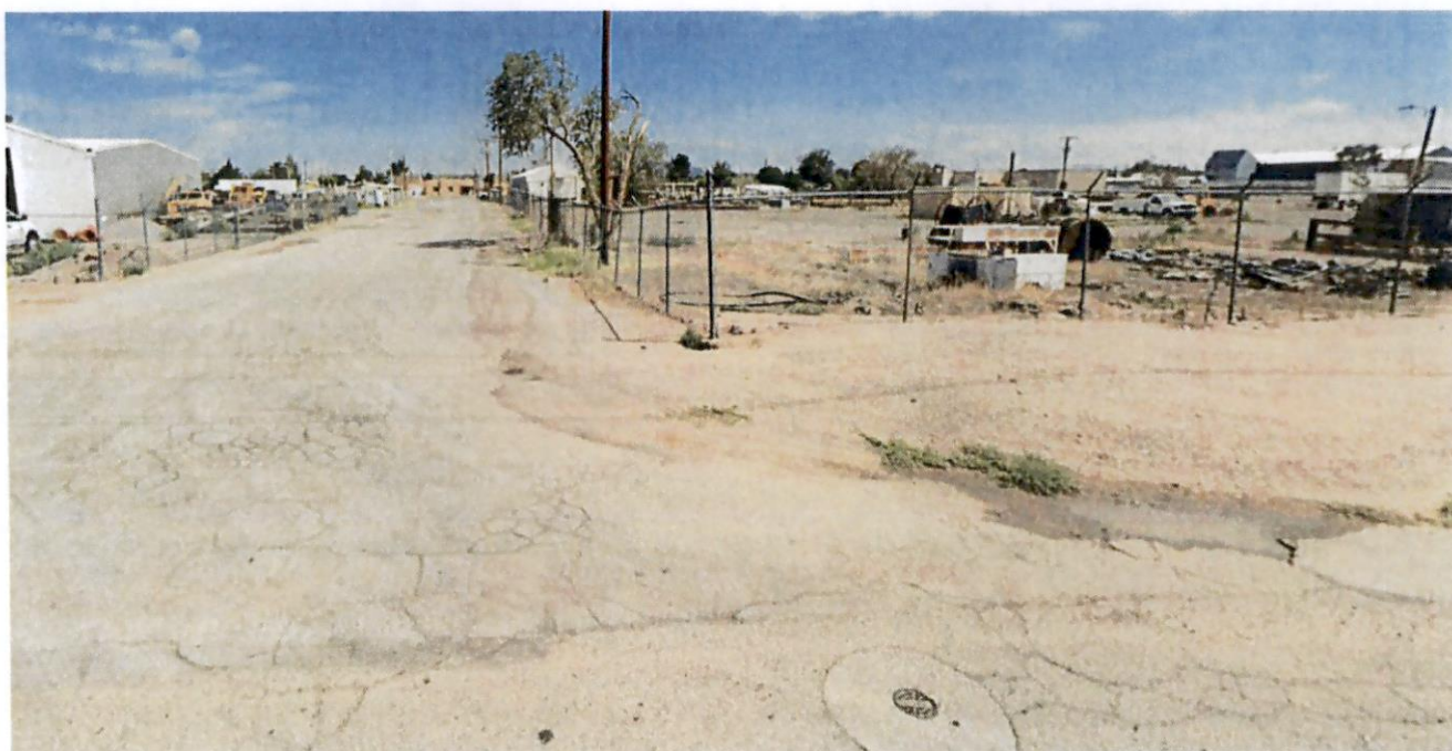
Appendix Image 3. Deteriorating street conditions in Amador Proximo and South area.
