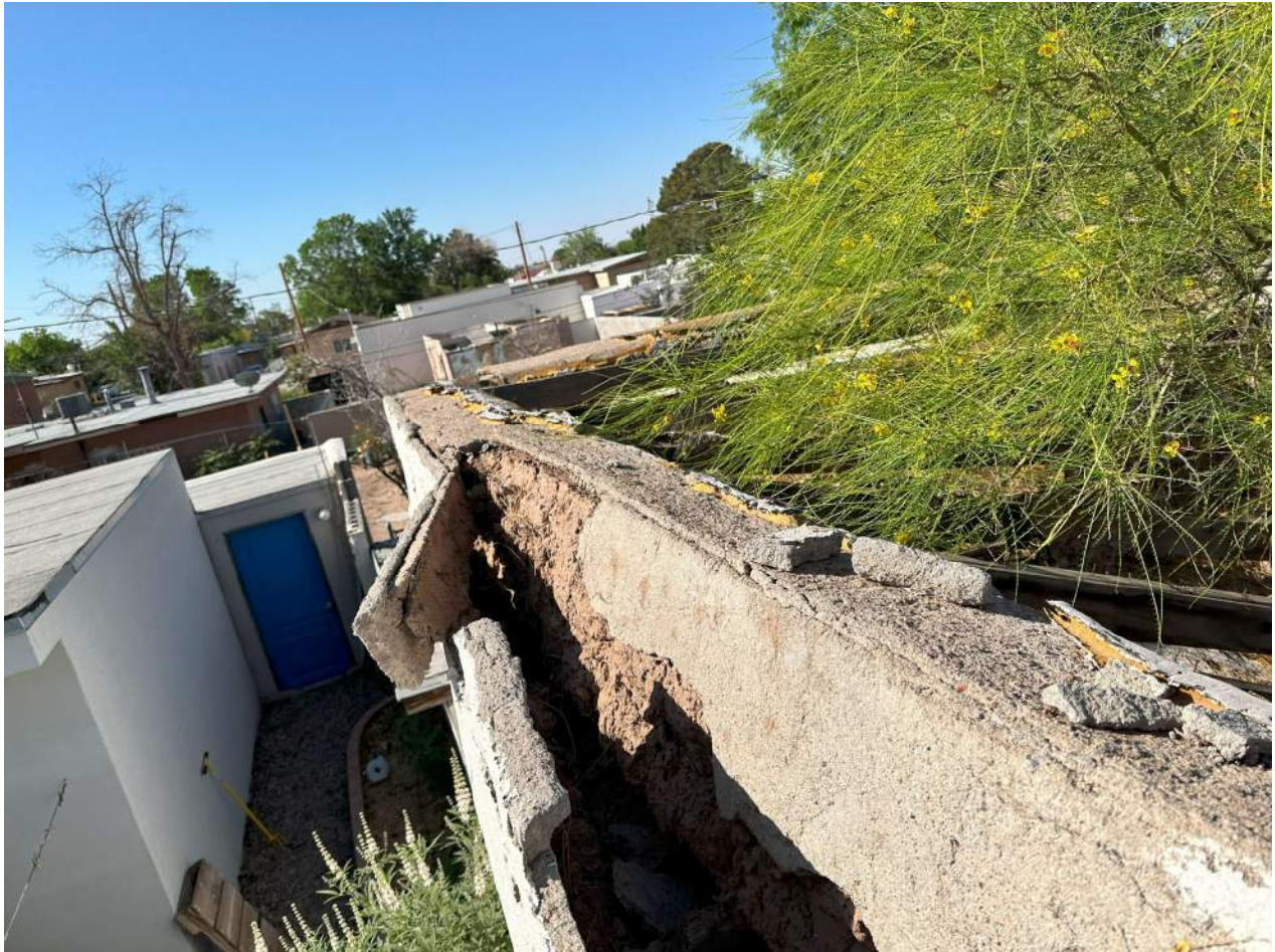
Photo 4 West unit wall, significant deterioration
