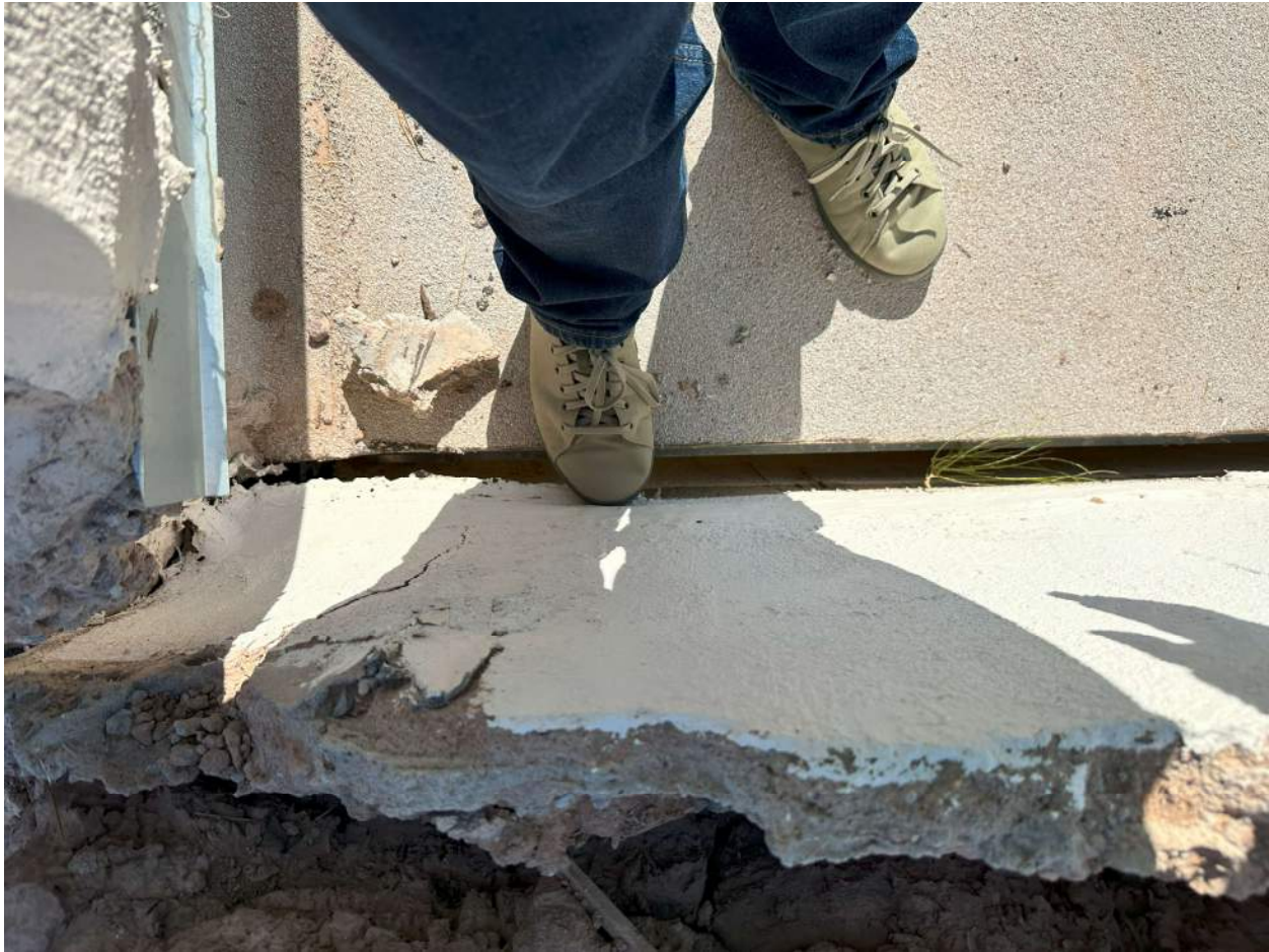
Photo 3 Gap between east unit patio and west unit
