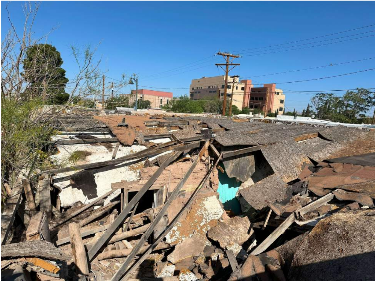
Photo 2 West unit, roof collapsed.
