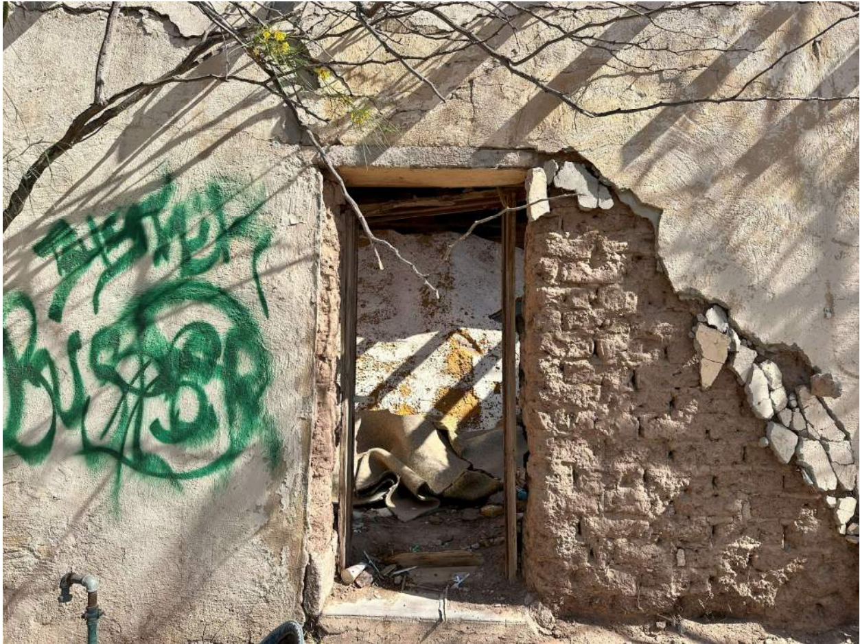
Photo 10 Rear of west unit, wall deteriorating
