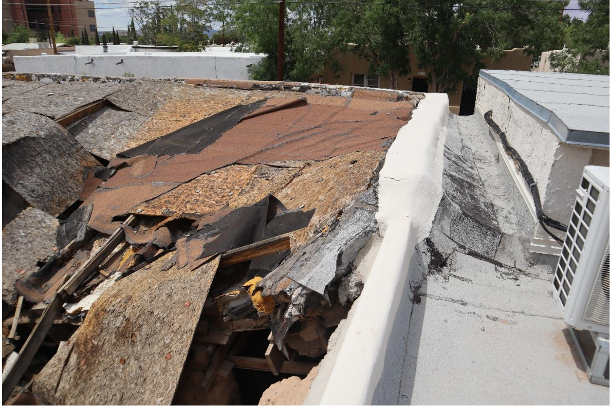
Figure 4:Roof of party wall between 422 E. May and 414 E. May. Photo taken July 1, 2025.
