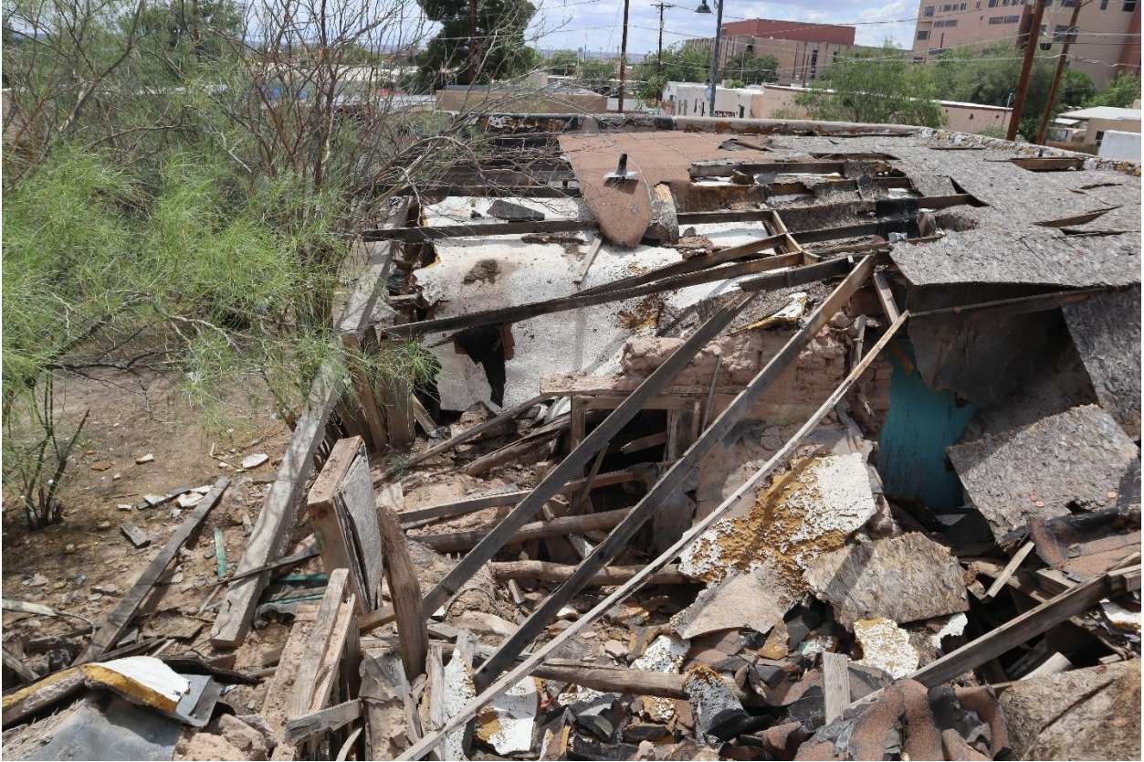
Figure 14: Photo of Collapsed roof, south facade at 414 E. May. Photo taken July 1, 2025.
