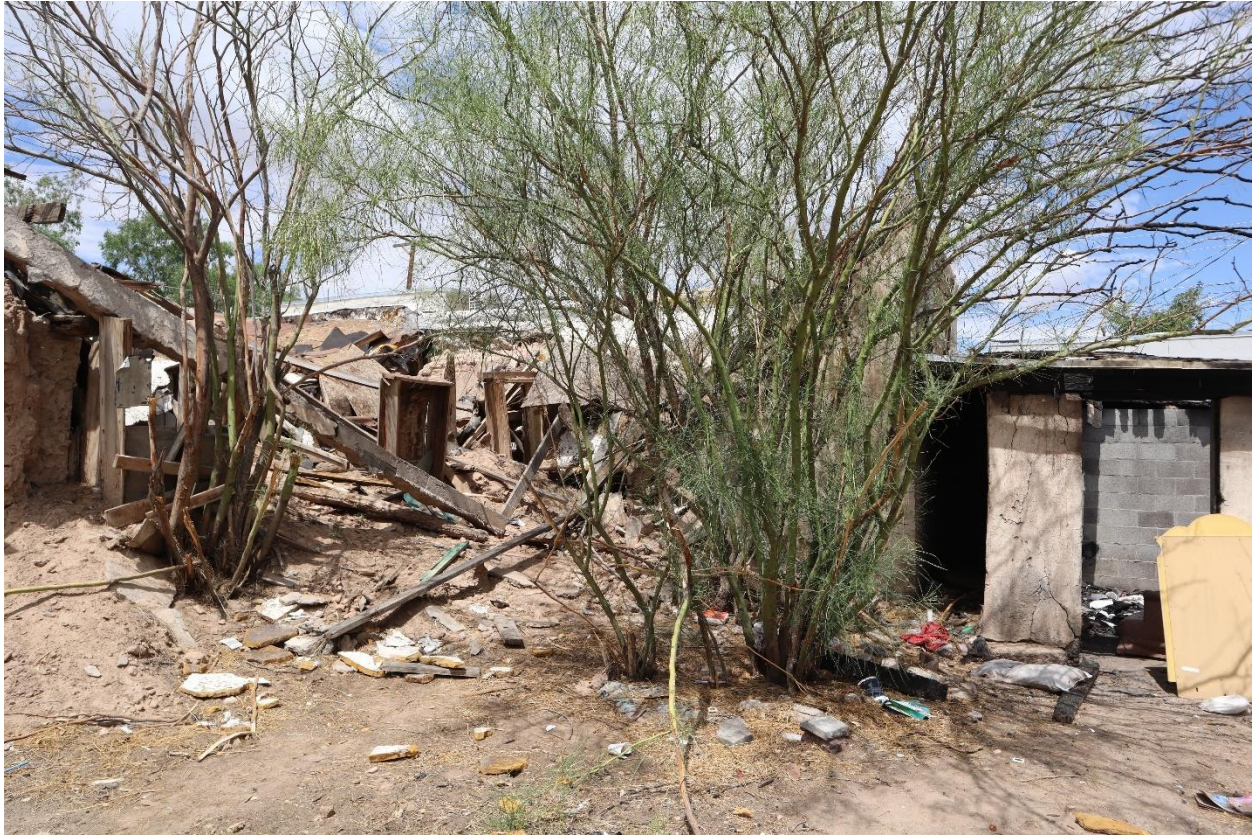
Figure 9: Collapsed roof and melted adobe mix on south façade of property. Photo taken July 1, 2025.
