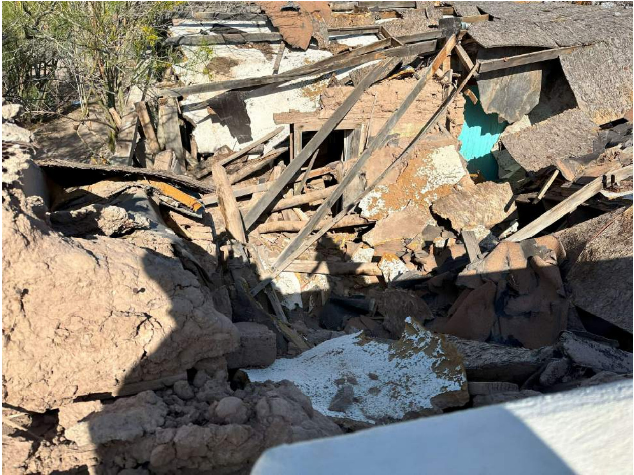
Photo 1 West unit, roof collapsed.
