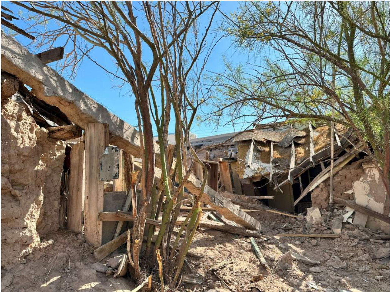
Photo 8 Rear of west unit, walls and roof collapsed
