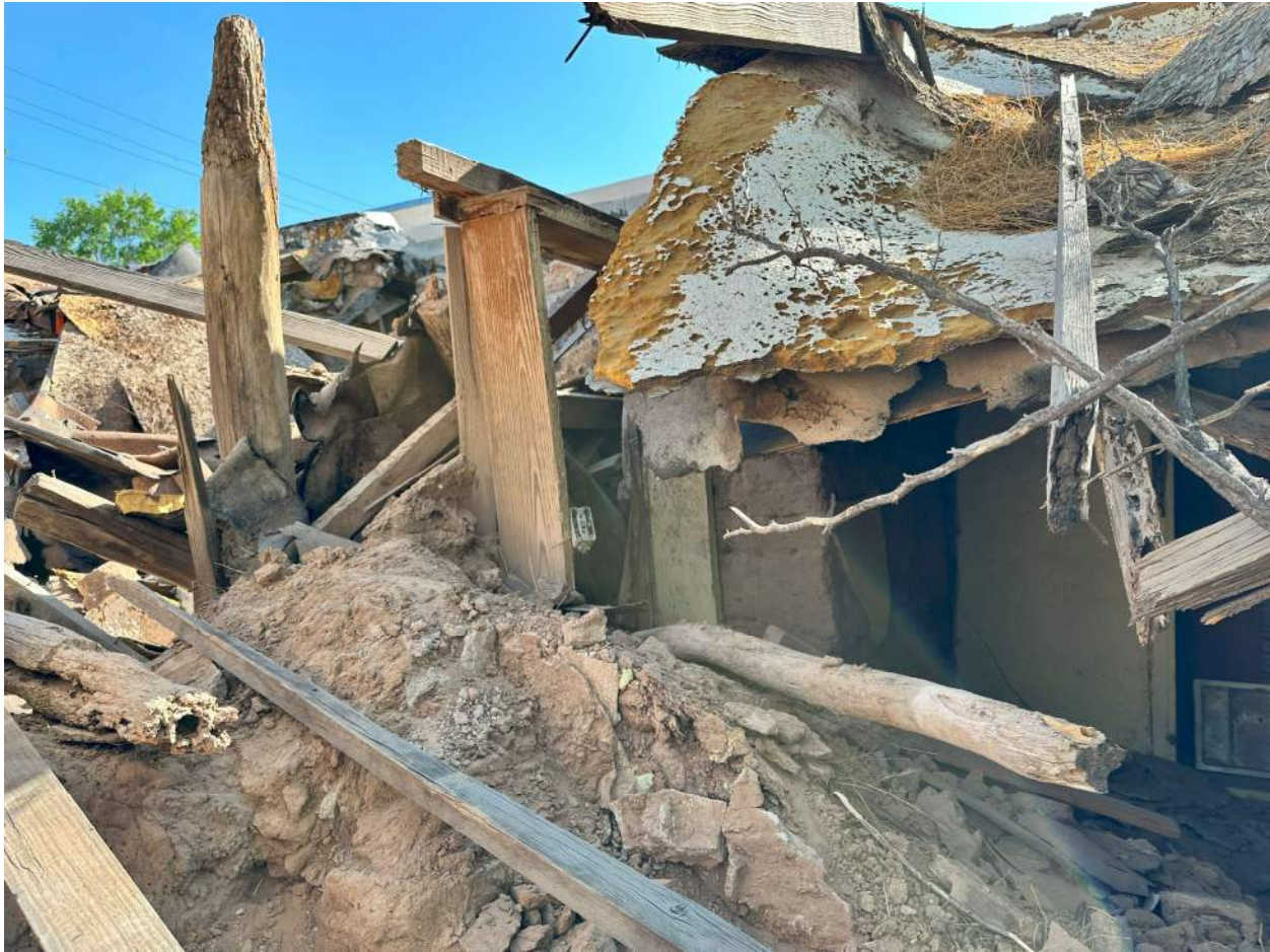
Photo 9 Rear of west unit, roof and walls collapsed.
