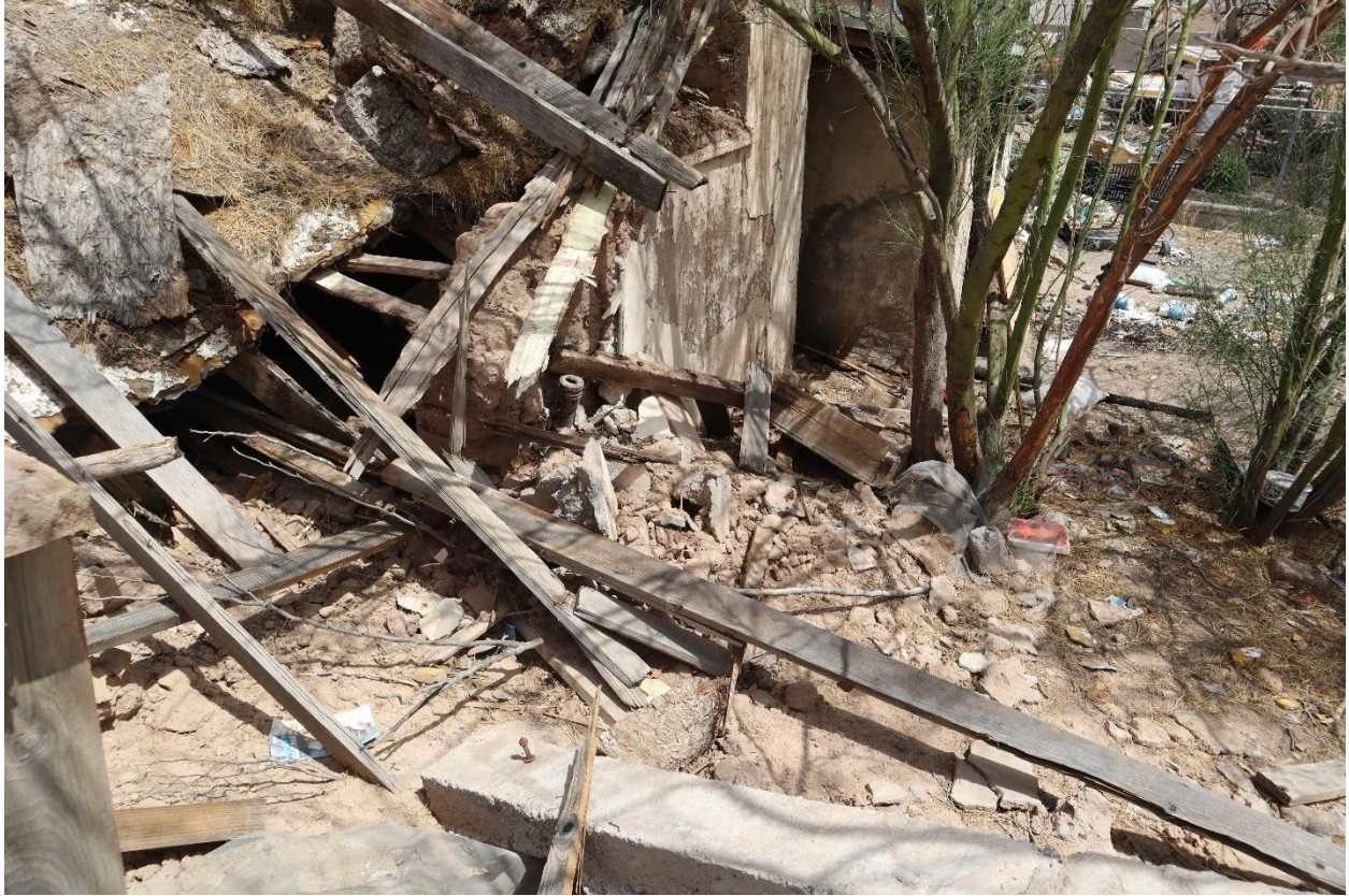
Figure 11: Detail of collapsed roof and wall structure. Photo taken July 1, 2025.
