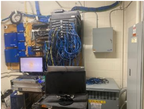
Electrical and IT
