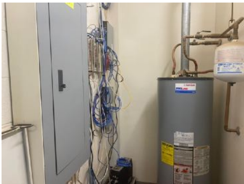
Electrical / IT / Mechanical Room
