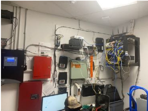
Existing Wing – Electrical / IT
