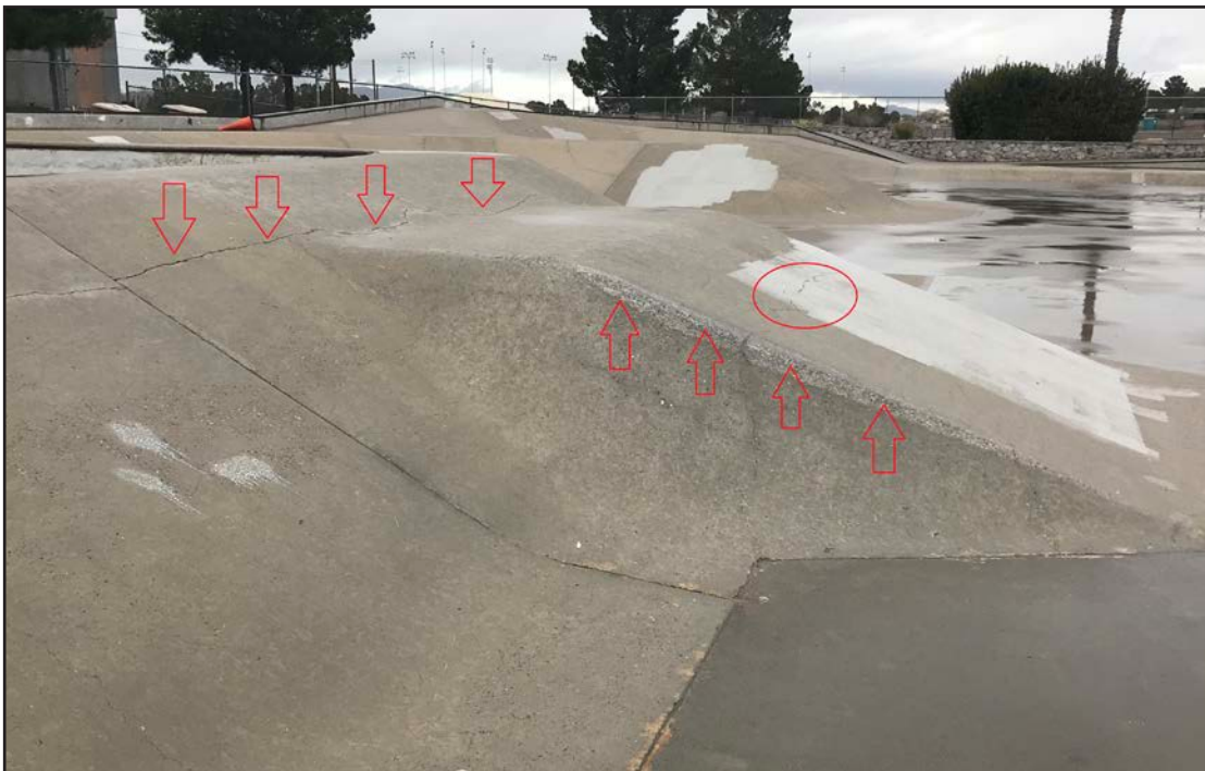
Feature #15 (low speed) - Low Bank: The bank has exposed concrete edges that are starting to reveal the aggregate and cause an inconsistent riding surface. The surface area is also showing spalling/cracking that could possibly impede the riders momentum.
