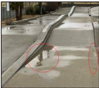
Water Pooling & Cracked Concrete
