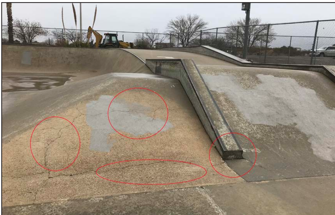
Feature #1 (low speed) - Half Pyramid w/Ledge: This feature is showing signs of concrete spalling/cracking on the surface and the toe/blend of the Half Pyramid is not smooth and has a kink at the bottom. The ledge height is also too steep and too short in order to properly land a trick.
