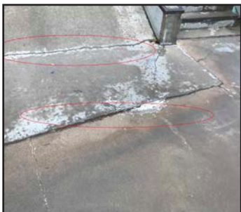
Spalling/Cracking & Large Cold Joint
