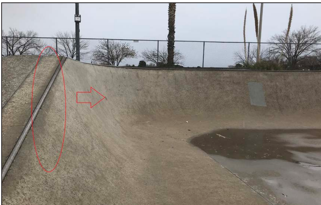
Feature #2 (high speed) - Bowled Corner: The coping reveal at the edge appears to be sunken into the concrete, which does not provide an adequate grind or slide for the rider. The coping reveal is also inconsistent as it wraps around the corner of the bowl which can be misleading for a rider.
