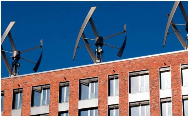
Energy production through roof mounted wind turbines
