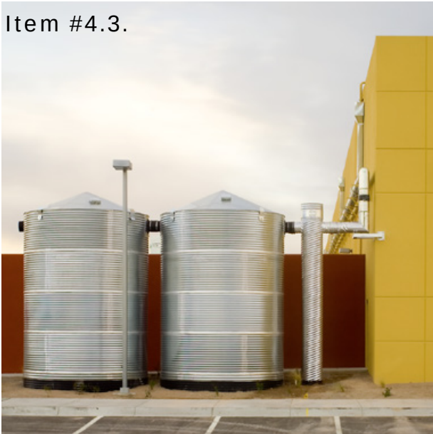
Cisterns to capture runoff from building roofs
