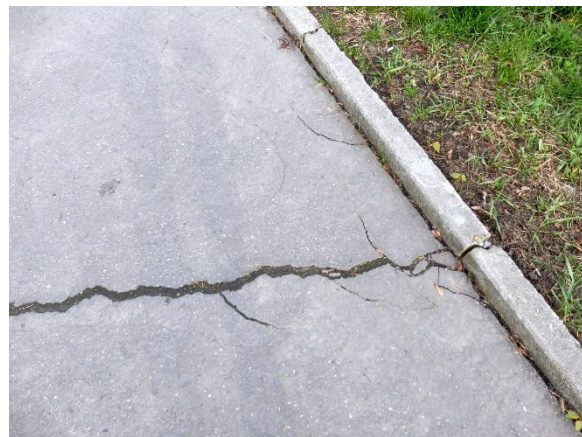
Example of Sidewalks Damaged by Construction Activity
