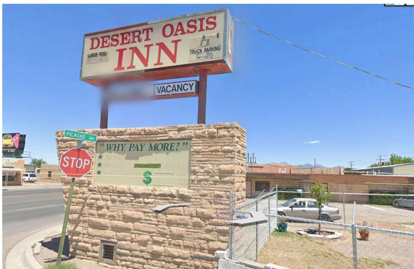
Image 21. Deteriorated and outdated signage on motel buildings.
