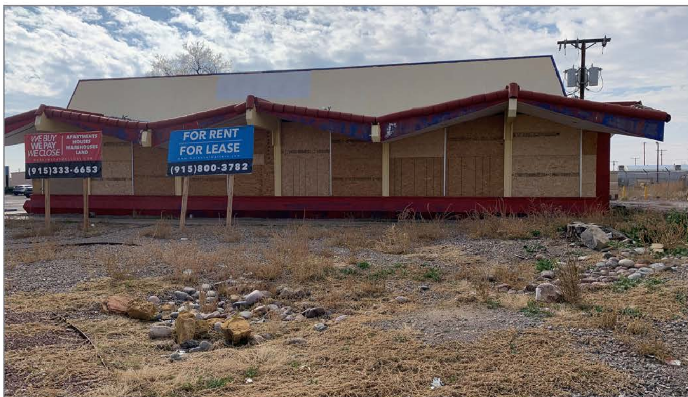
Image 8. Building on Main St. in need of roof replacement and other rehabilitation.
