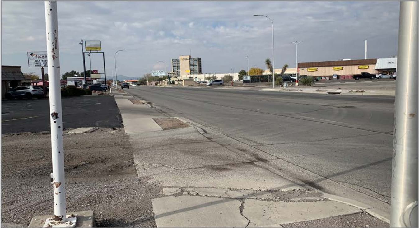
Image 13. Extensive deterioration of sidewalks along El Paseo Rd.
