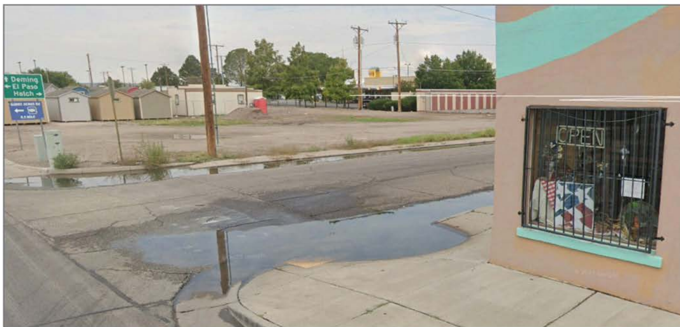
Image 22. Drainage issues leading to pooling along West Picacho Ave.
