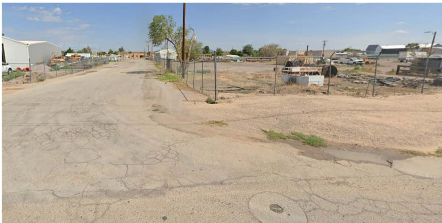
Appendix Image 3. Deteriorating street conditions in Amador Proximo and South area.
