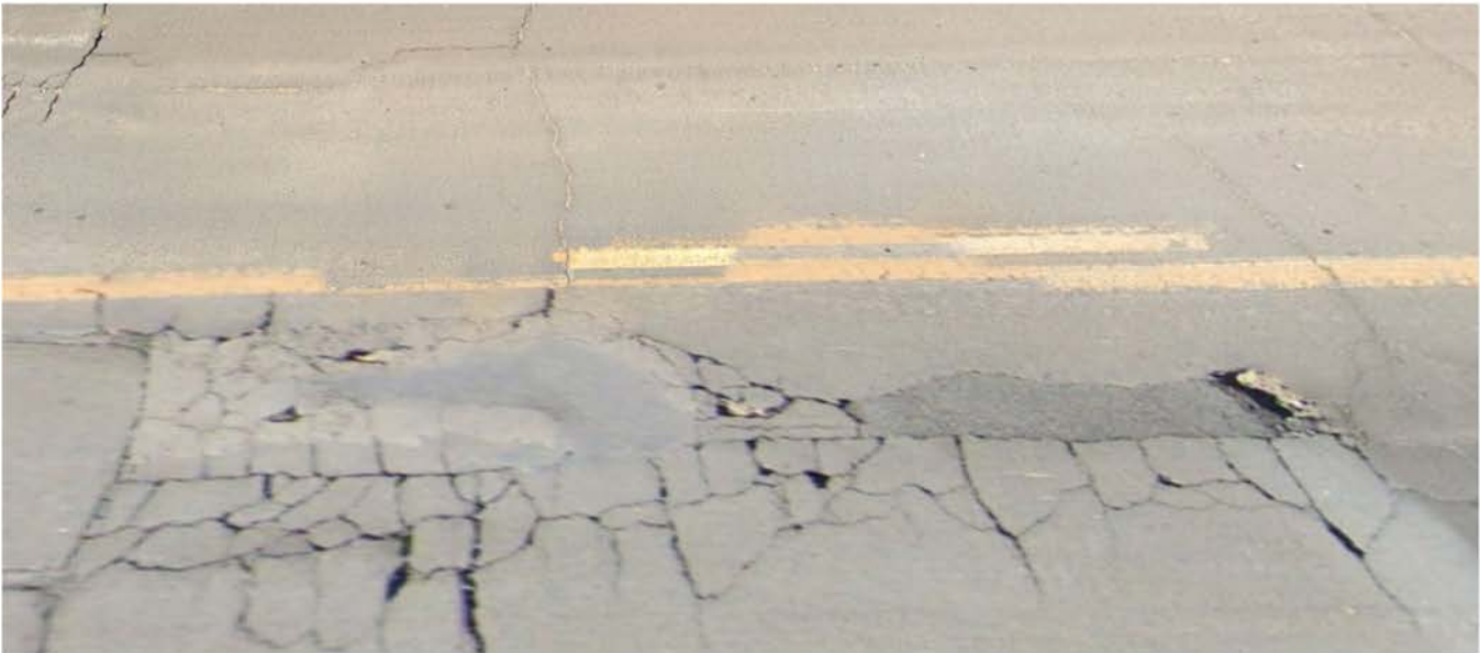
Image 12. Deteriorating pavement along South Solano Dr.
