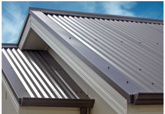
Corrugated metal roofs with exaggerated seams are not appropriate for the Las Cruces historic districts.
