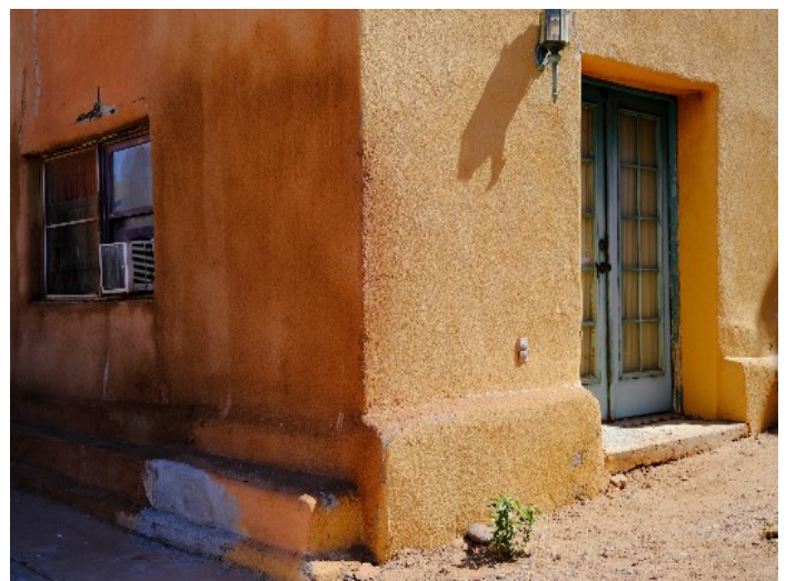
The addition of concrete "collars" can cause moisture and cracking issues and is not approvable for adobe buildings. Adobe building with multiple collars (Mesquite Original Townsite Historic District).
