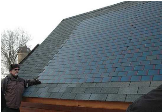
Solar shingles appropriately mounted on a rear roof line (above).
